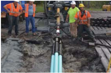
Tideland Electric Cooperative Bellhaven, NC
