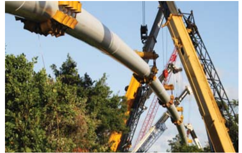
Florida Power & Light Company St. Lucie, FL
