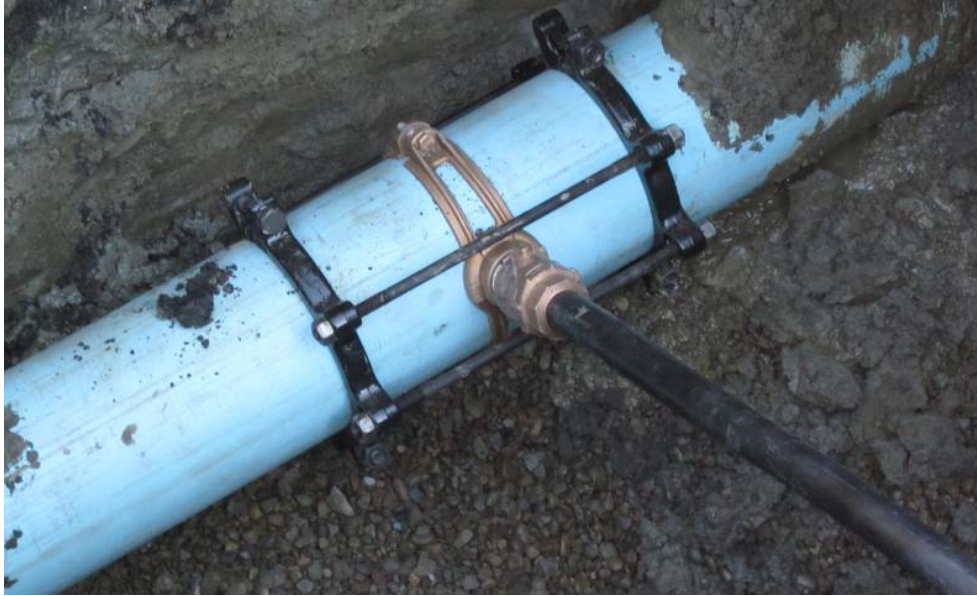
Figure 7. Service saddle installation showing the use of the bell restraint harnesses for axial stress management at the tap location.
