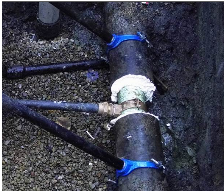
Figure 8. Typical service saddle connection on 6-inch force main and grout venting lines on existing cast iron line.
