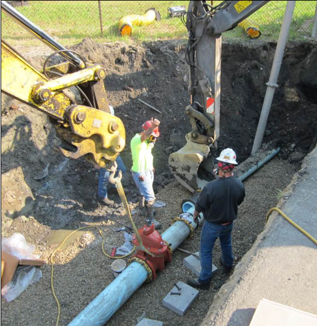
Figure 6. Typical fire hydrant installation and HDD pipe section tie in inside entry/exit pit location.
