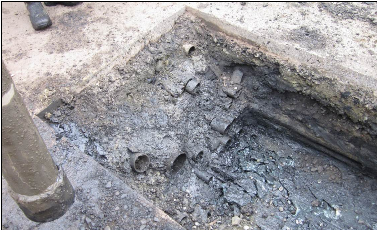
Figure 3. Explorative excavation showing contaminated soils and existing utilities, including a multitude of process lines.
