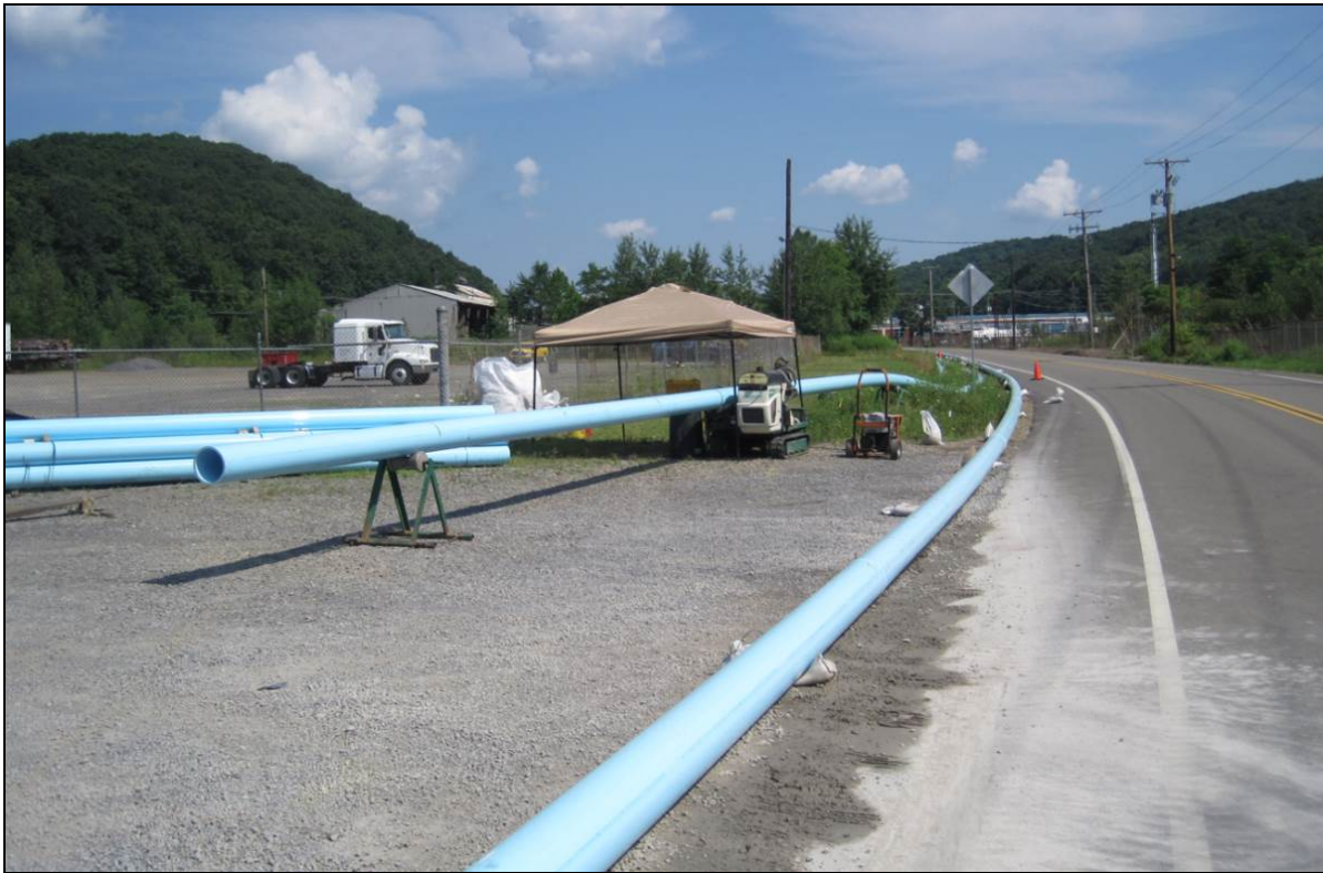
Figure 4. Fusion staging and assembly layout for the waterline to be installed using HDD methods.
