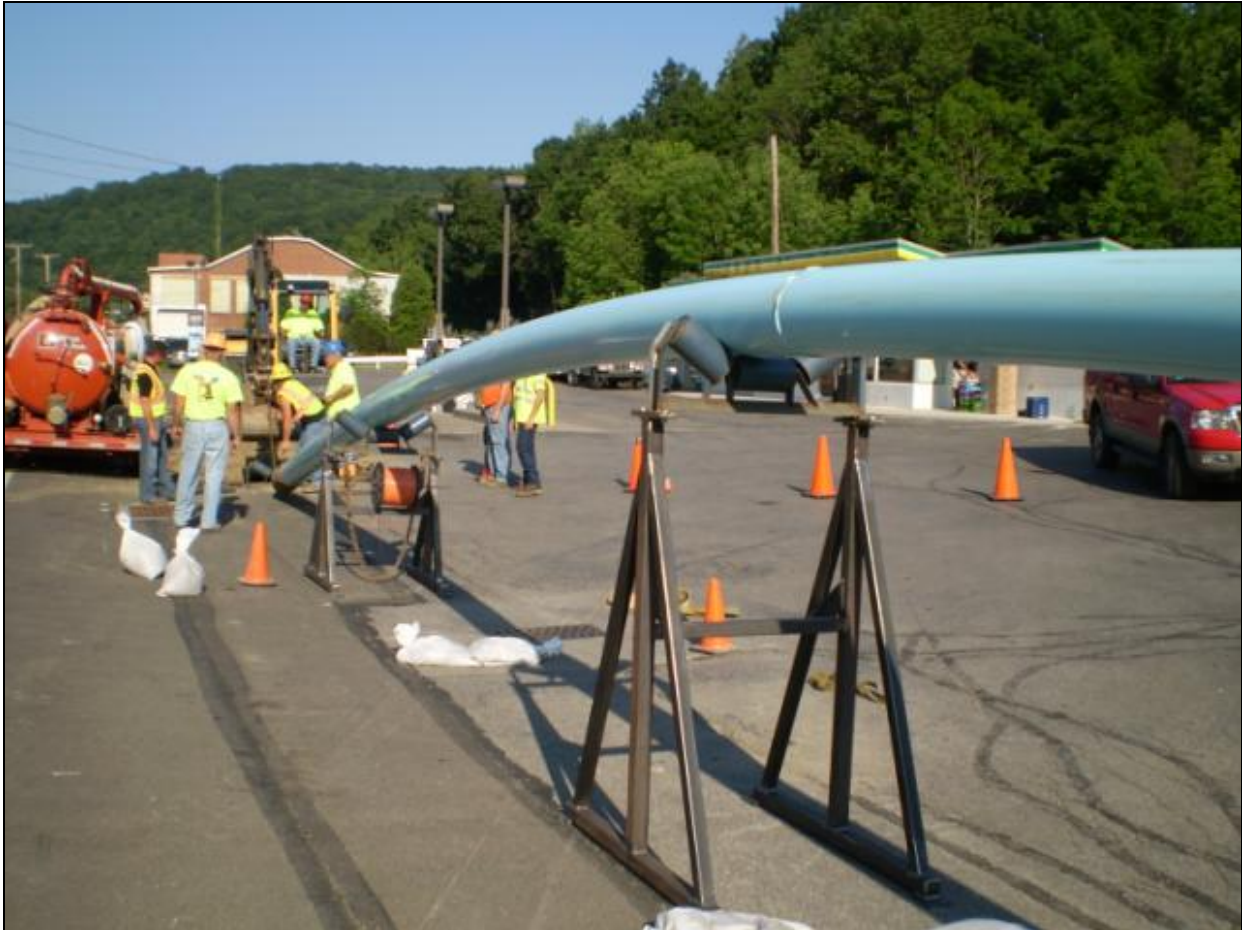
Figure 5. Typical insertion location for the HDD entry pit, illustrating the “abbreviated aerial entry” method.
