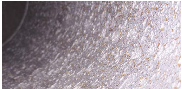
Pitting before cleaning and coating
